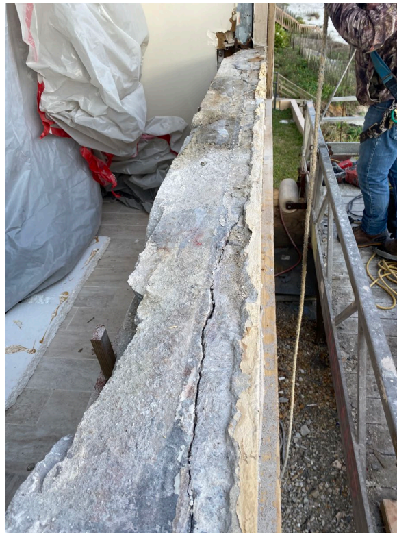
Picture 2: Cracked window sill of Unit 102
